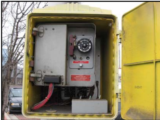
Pictured Above: Electro-Mechanical controller type Picture at Right: Eagle/EPAC 300 controller type
